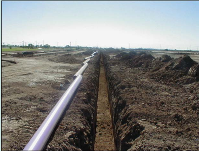
Reclaimed water pipeline, City of Chandler
