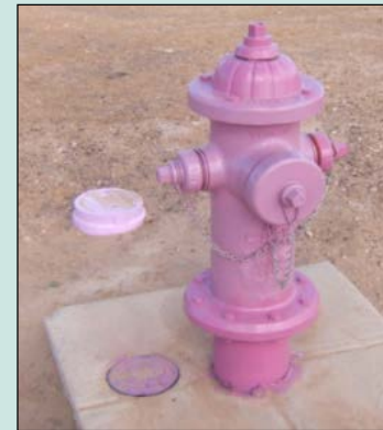
Reclaimed Water Fire Hydrant
